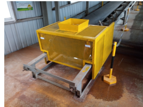
整改后的皮带机尾部防护罩 Protection cover at rear of conveyor after rectification
